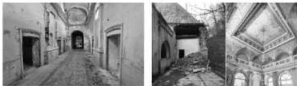
Figure 5. Băile Neptun degradation situation
